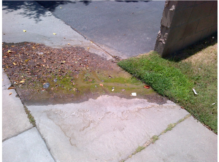
This broken sprinkler is not doing its job, wastes precious water and is helping to move any contaminants offsite and into surface water.
